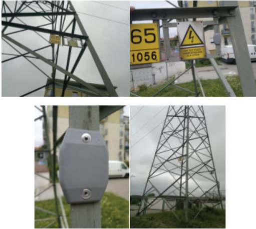
Figure 3. RFID tag installed on HV pole
