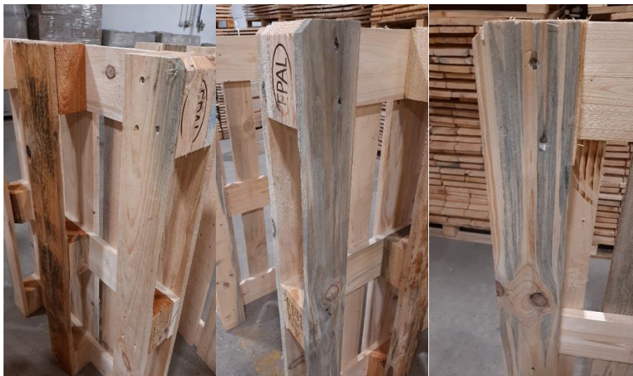
Figure 7. Discolouration, staining Source: own elaboration.
